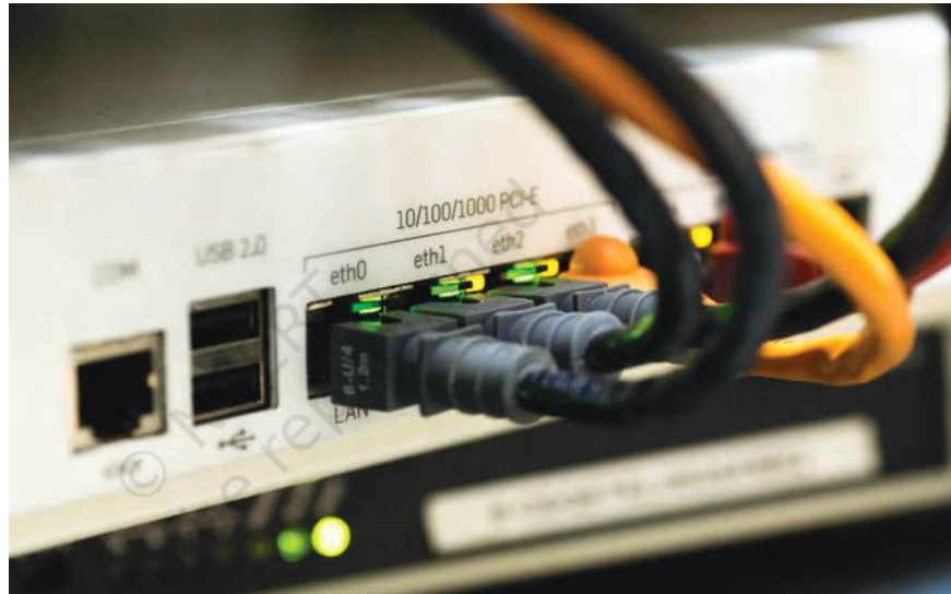
Figure 5.9: Cables connected to a network switch
