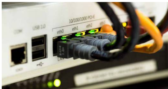
Figure 10.12: Cables connected to a network switch
