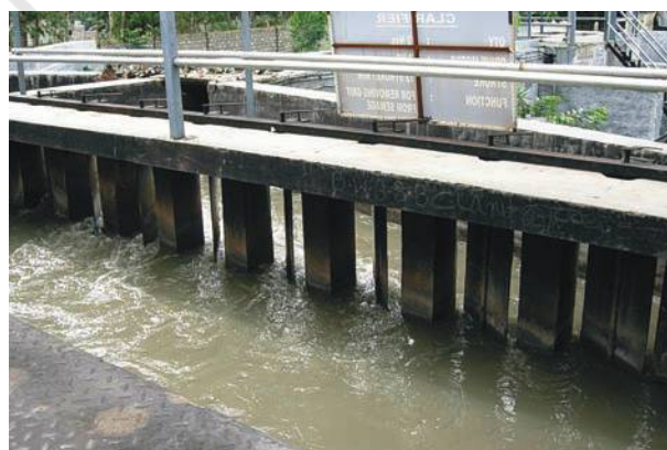
Fig. 18.4 Grit and sand removal tank
